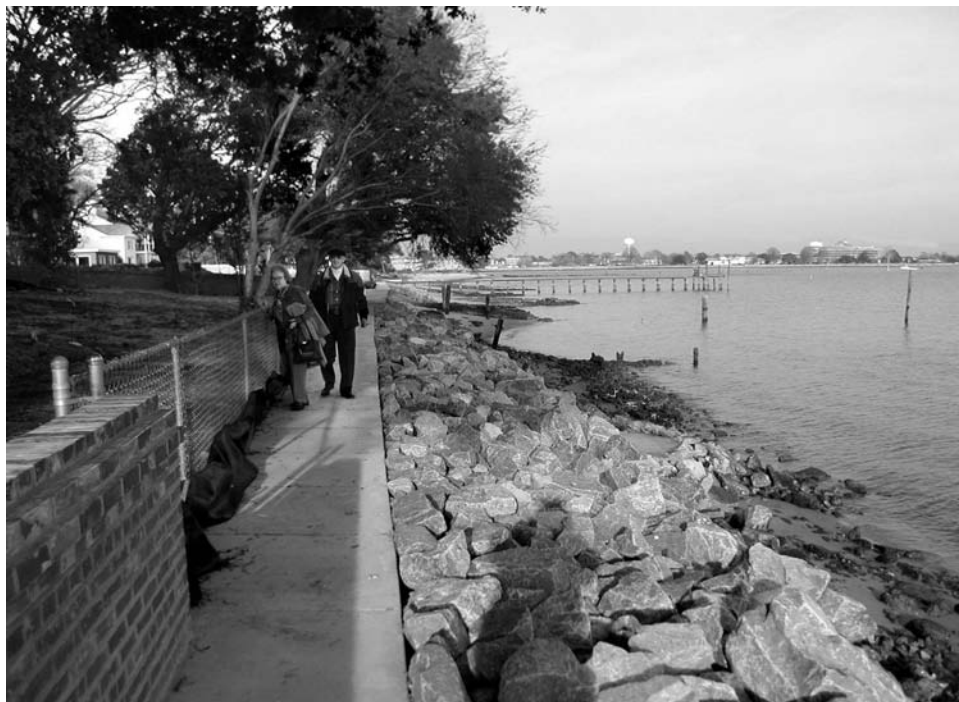
McDonald's waterfront repairs: new seawall, brick wall, fence, and sidewalk. Photo by W. Przypek.
